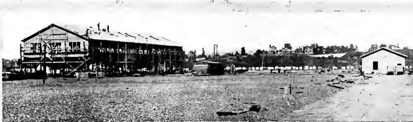
Work progressing on the site of the Coast Shipbuilding Company's plant at Portland, Oregon.
